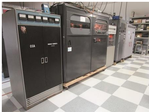
A portion of the collection's 15-transmitter lineup. The 2.5 kW CCA “cow killer” is at the extreme left.
