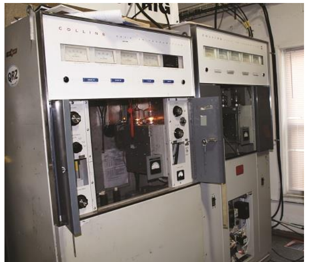
Two of Moersdorf’s set of five Collins 20V Series of 1 kW rigs. All have been modified for use on the amateur radio 40-, 75- and 160-meter bands.
